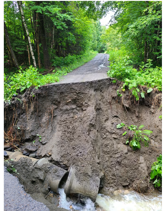
Dubray Road damage.
