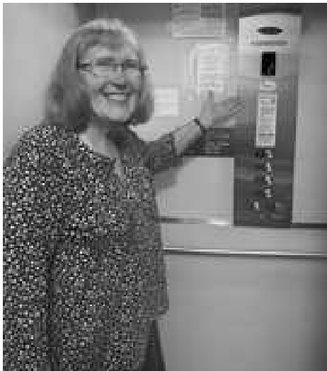
Betty showing off new lift control panel.
